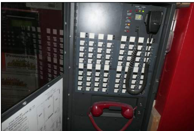
Photo 107 Fire Protection Systems
