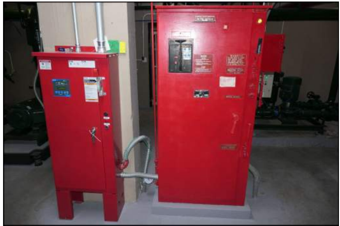
Photo 100 Fire Protection Systems
