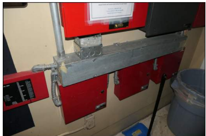
Photo 108 Fire Protection Systems
