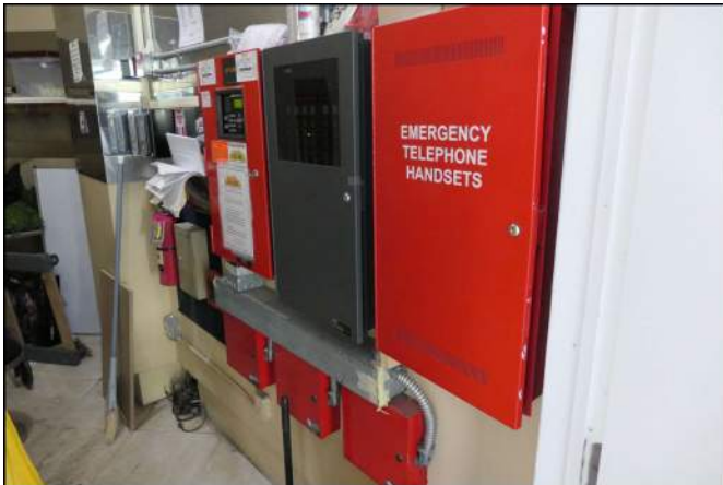
Photo 111 Fire Protection Systems
