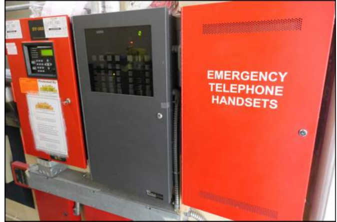
Photo 104 Fire Protection Systems
