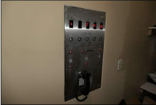
Photo 109 Fire Protection Systems
