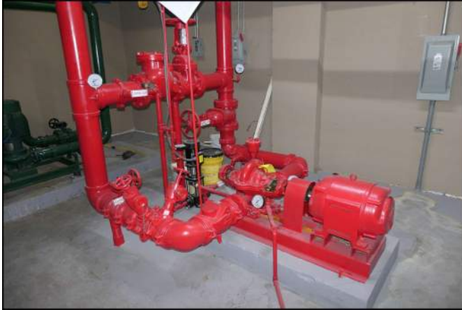
Photo 97 Fire Protection Systems
