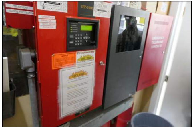
Photo 112 Fire Protection Systems
