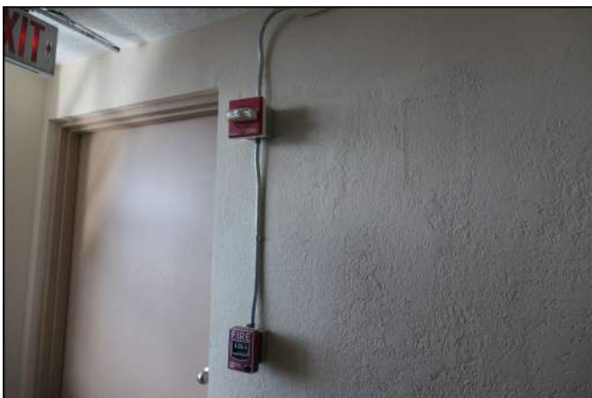
Photo 113 Fire Protection Systems
