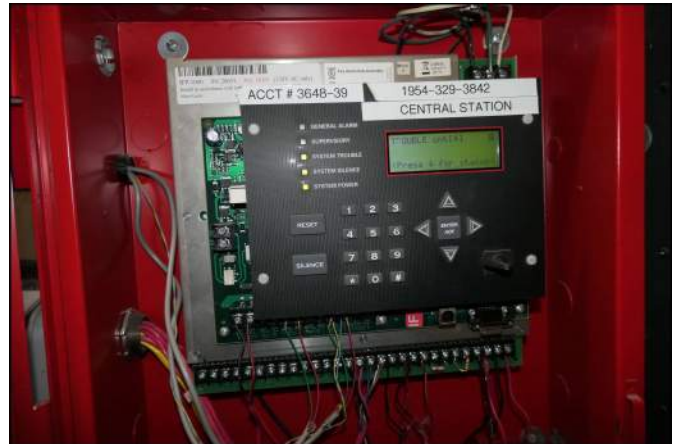
Photo 106 Fire Protection Systems
