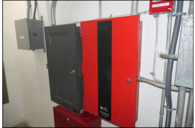
Photo 110 Fire Protection Systems
