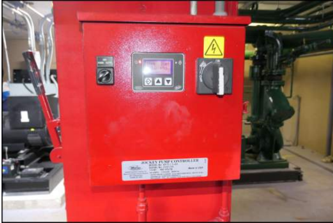
Photo 103 Fire Protection Systems
