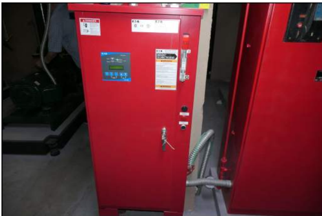
Photo 101 Fire Protection Systems
