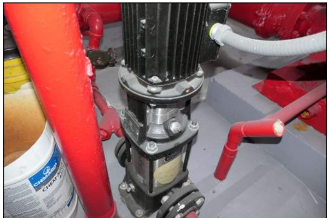
Photo 102 Fire Protection Systems
