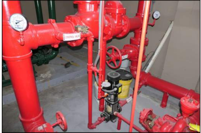
Photo 98 Fire Protection Systems
