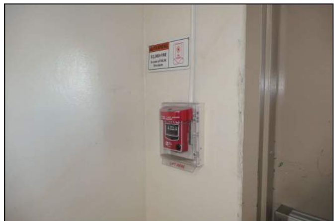
Photo 114 Fire Protection Systems
