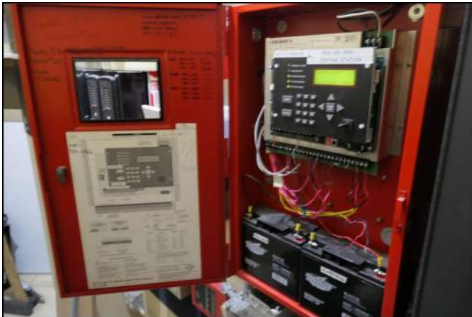
Photo 105 Fire Protection Systems
