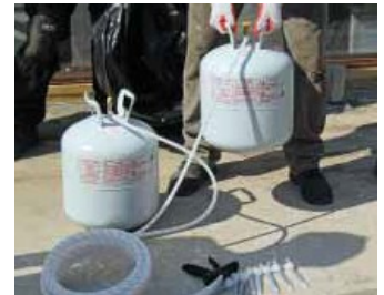
Shaking of A-side and B-side tanks
